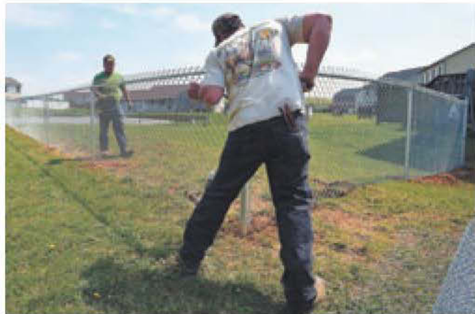
A two-man crew from Horst Fencing completes a new fence installation by stretching a chain-link section, which is available in silver, black, brown and green.
